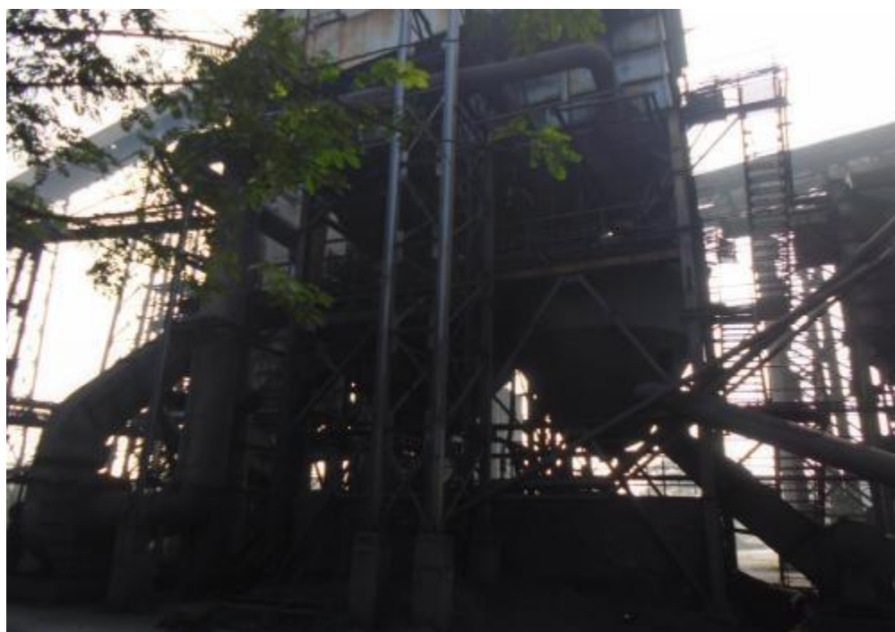
(figure 8: DRI New Bagfilters - Cap:33,200 m 3 /hr)
